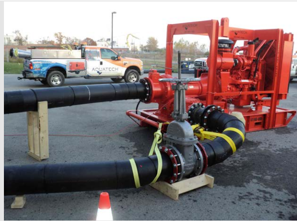
Pump showing Suction and Discharge Piping
