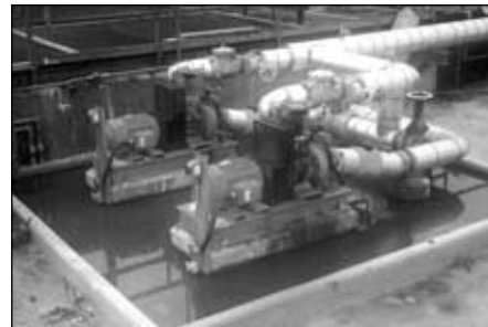
API Separator Sludge Removal – Permanent installation of two 6" (150mm) CD150M electric drive Dri-Prime pumps
