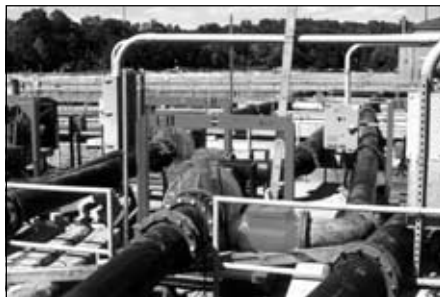
Wastewater Treatment Plant Bypass Project – Temporary installation of twelve 12" (300mm) DPC300 electric drive Dri-Prime pumps
