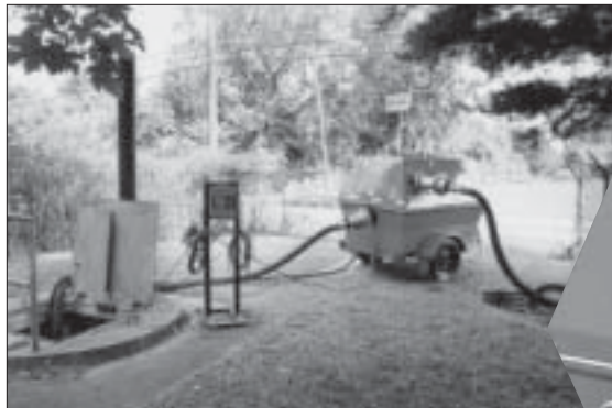
Municipal Pump Station Bypass
